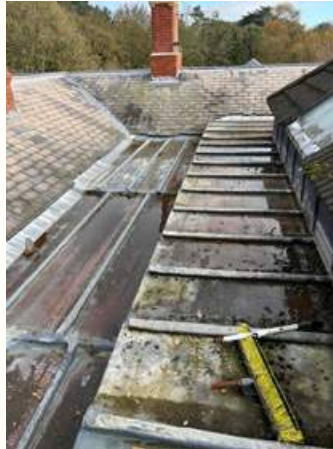
A - Ponding on flat lead roof.
