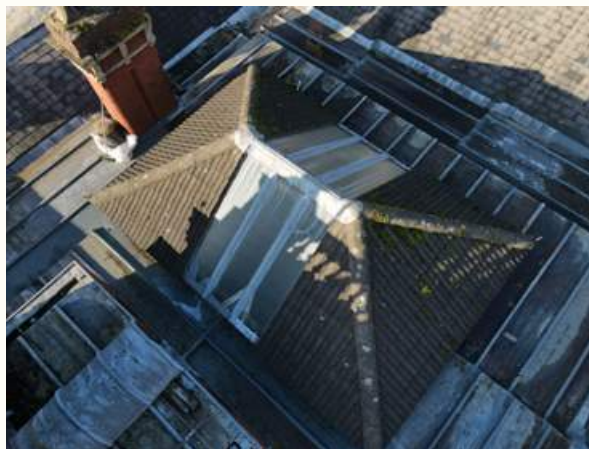
D - Damage to rooflight glazing.
