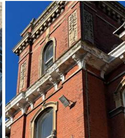
E - Damage to timber fascia.
