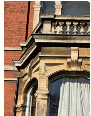
F - Stained/ damaged stonework.
