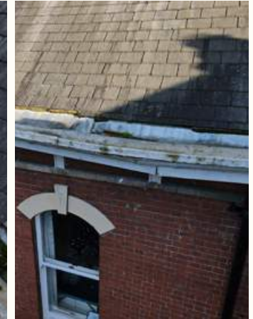
C - Damage to timber fascia.
